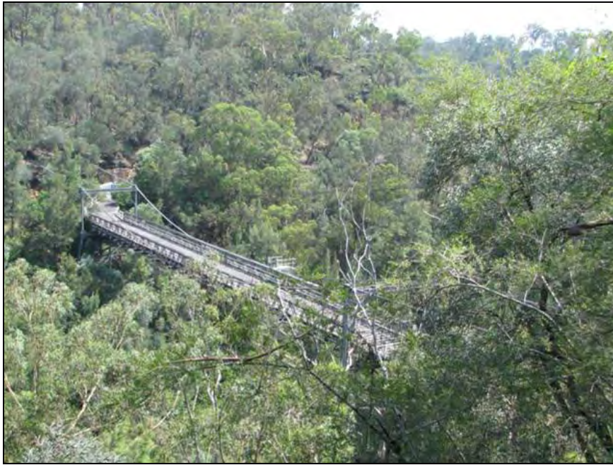
Plate 14 – 2011 photograph showing Maldon Suspension Bridge no longer in use (Source: Biosis Research).
